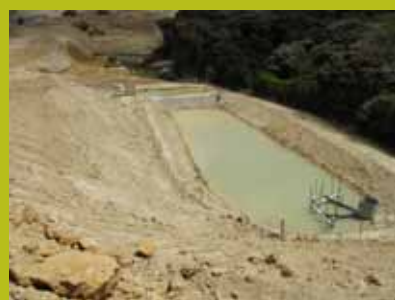
Sediment retention pond with flocculation, essential for sediment control at a subdivision within the Pauatahanui catchment
