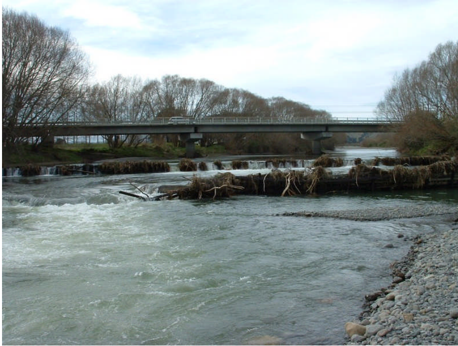
Photo 6: The failed Te Ore Ore grade control weir.
