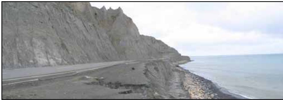
Figure 3: View south towards Whatarangi Bluff, showing extent of terracing required to achieve road platform
