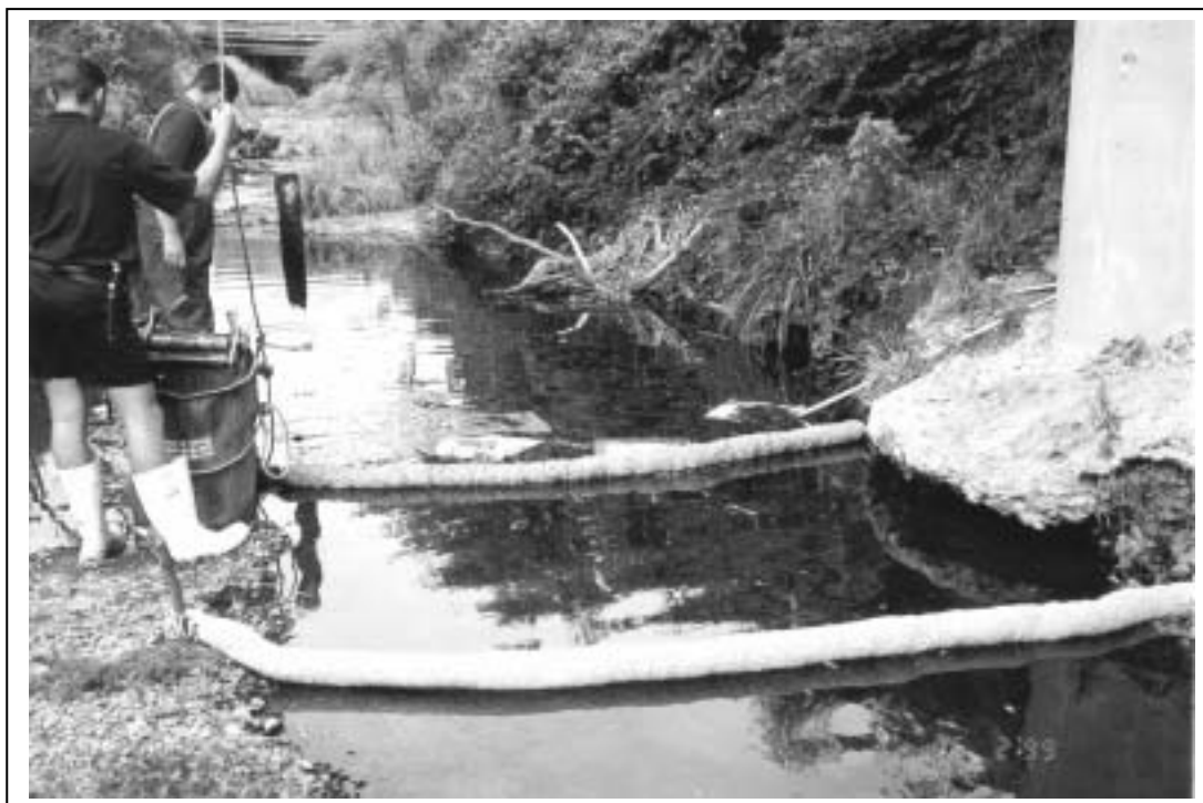
Figure 18: Clean up of an oil spill in the Porirua Stream on 16 February 1999. This spill occurred due to vandals overturning unsecured drums on a construction site.
