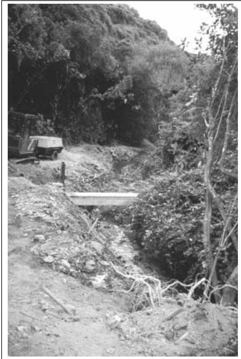
Figure 15: Unconsented works in the Kaiwharawhara Stream on 5 March 1999. Sediment from this work had effects over 2 kilometres downstream.
