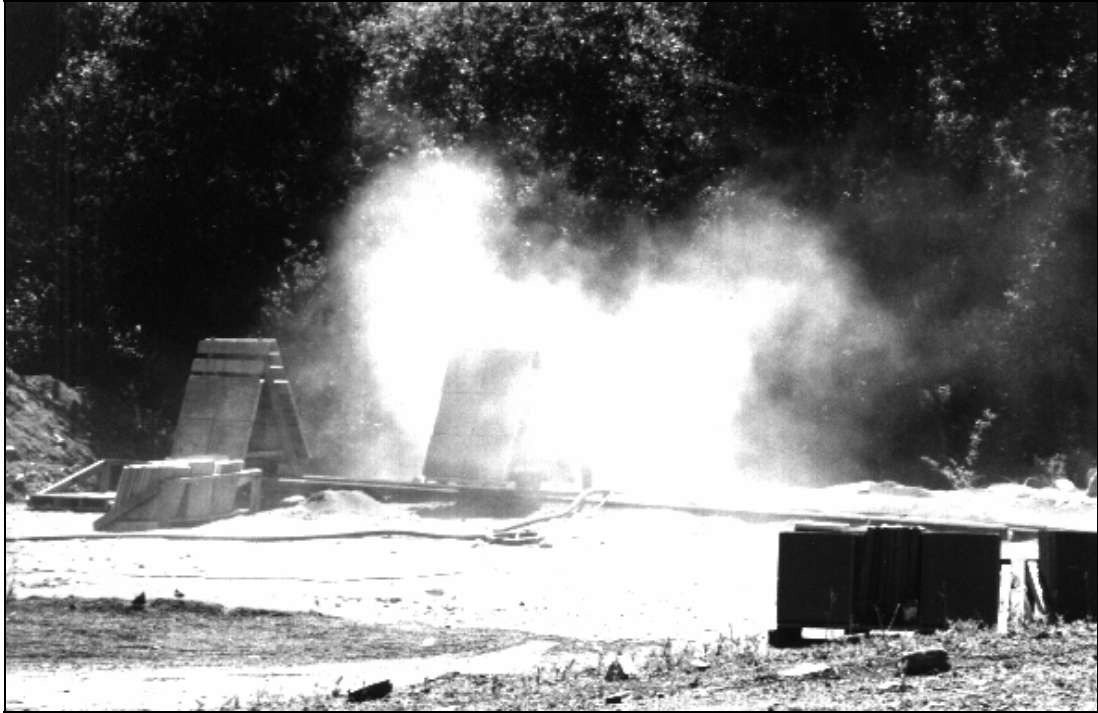
Figure 8: Dust from Wellington Concrete Products Ltd Undertaking Unconsented Dry Abrasive Blasting on 10 November 1997
