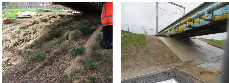
Figure 2: Erosion area and repair site under the Pomare Railbridge
