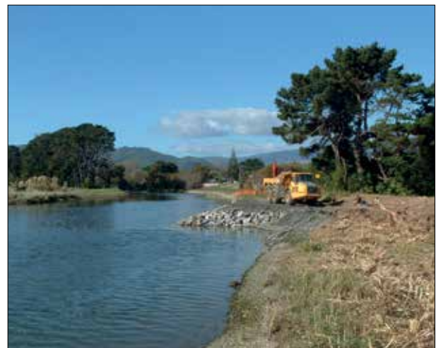
The management of the effects of flood protection activities is governed by the Code of Practice and resource consent conditions
