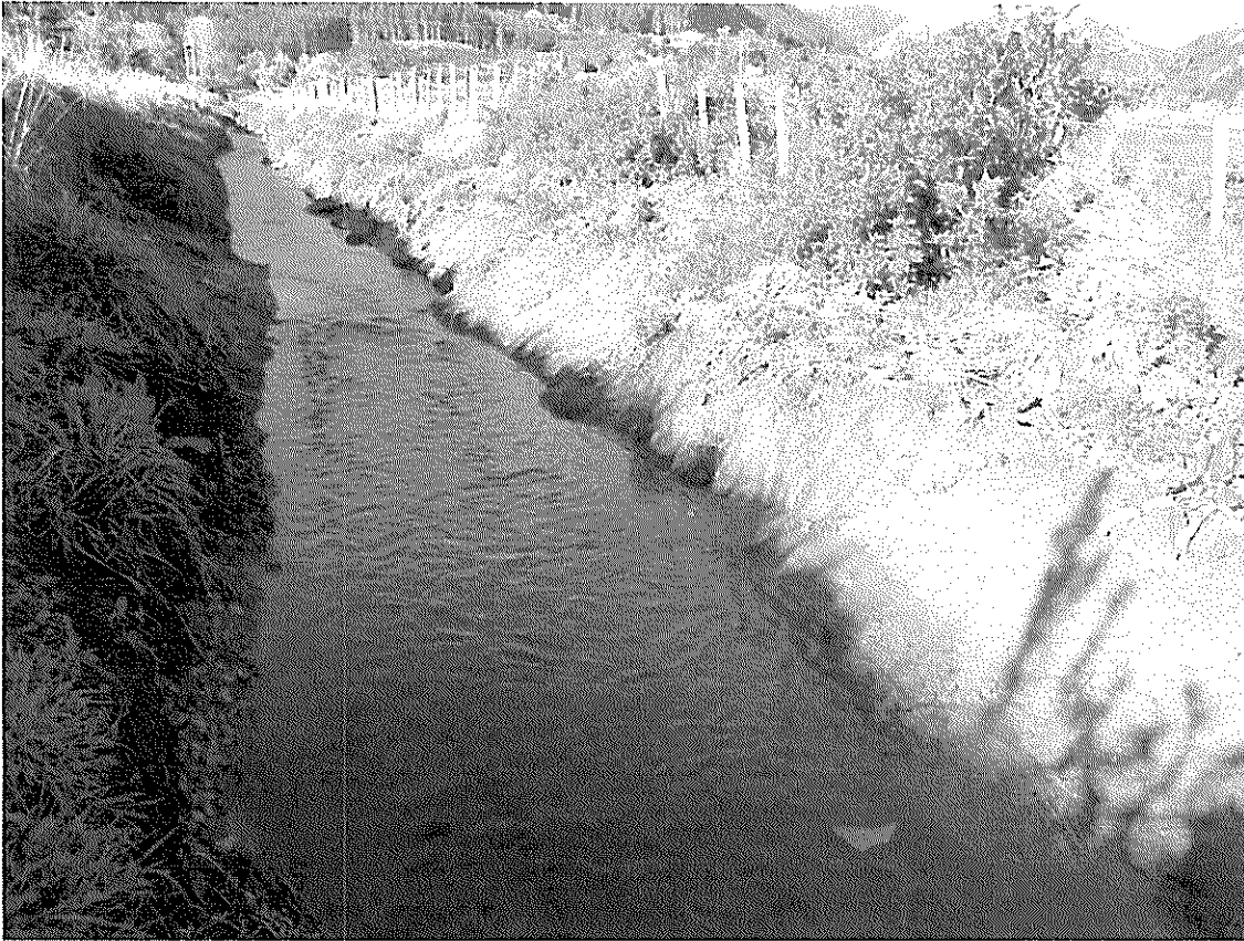
Illegal dredging May 2015. Carried out in the name of "drain clearing".
